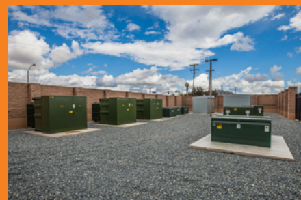
Moreno Valley Utility South Industrial Substation
