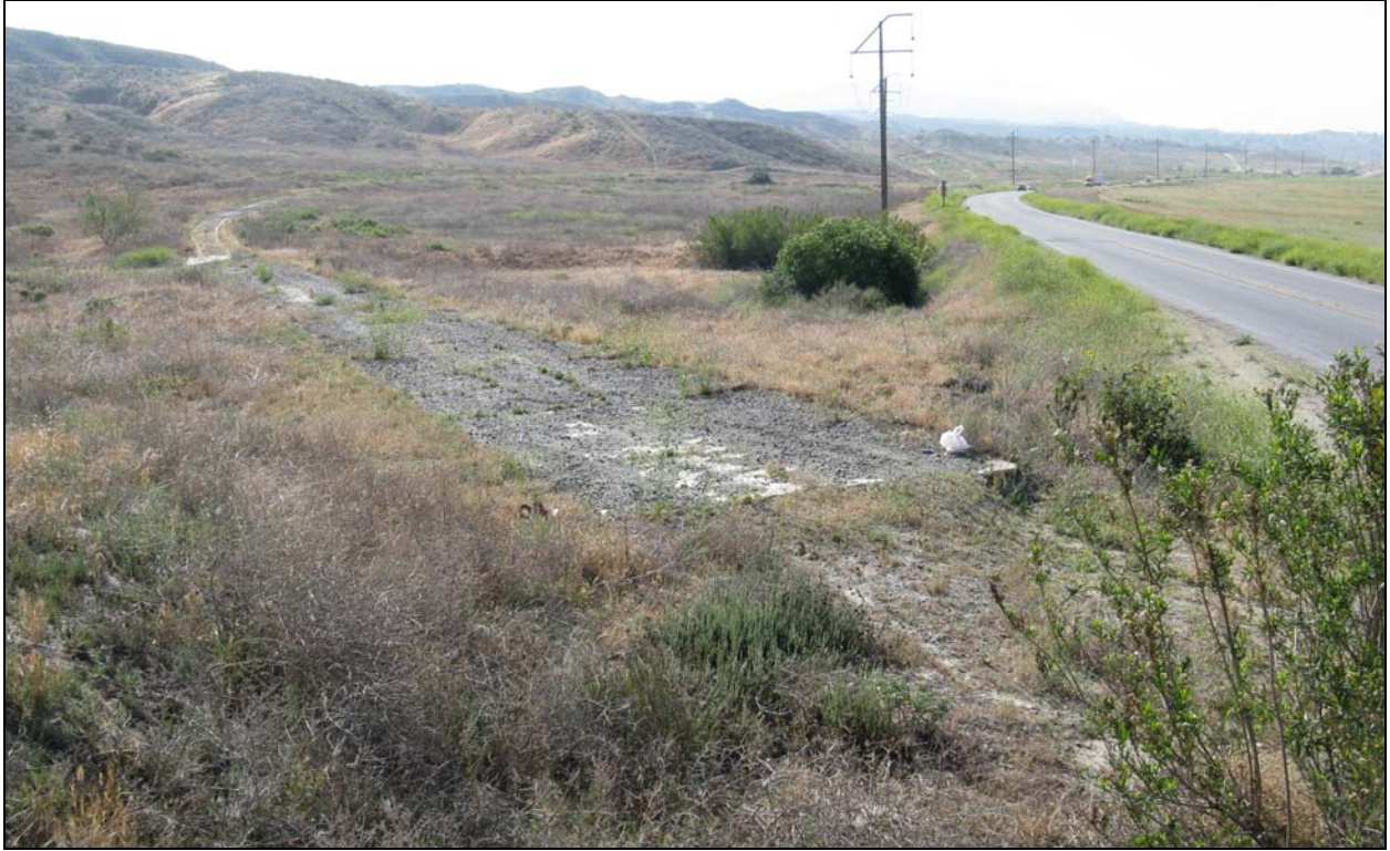
Figure 3. Abandoned segment of road found along Gilman Springs Road near the junction of Alessandro Boulevard (left-hand side of photograph; photograph taken May 9, 2012, view to the southeast). Note this segment measures 16 ft wide and is a 4-inch-thick concrete slab with a thin covering of gravel. This segment of road bed was once a curve at the juncture of Gilman Springs Road and Alessandro Boulevard that was abandoned by at least 1941.
