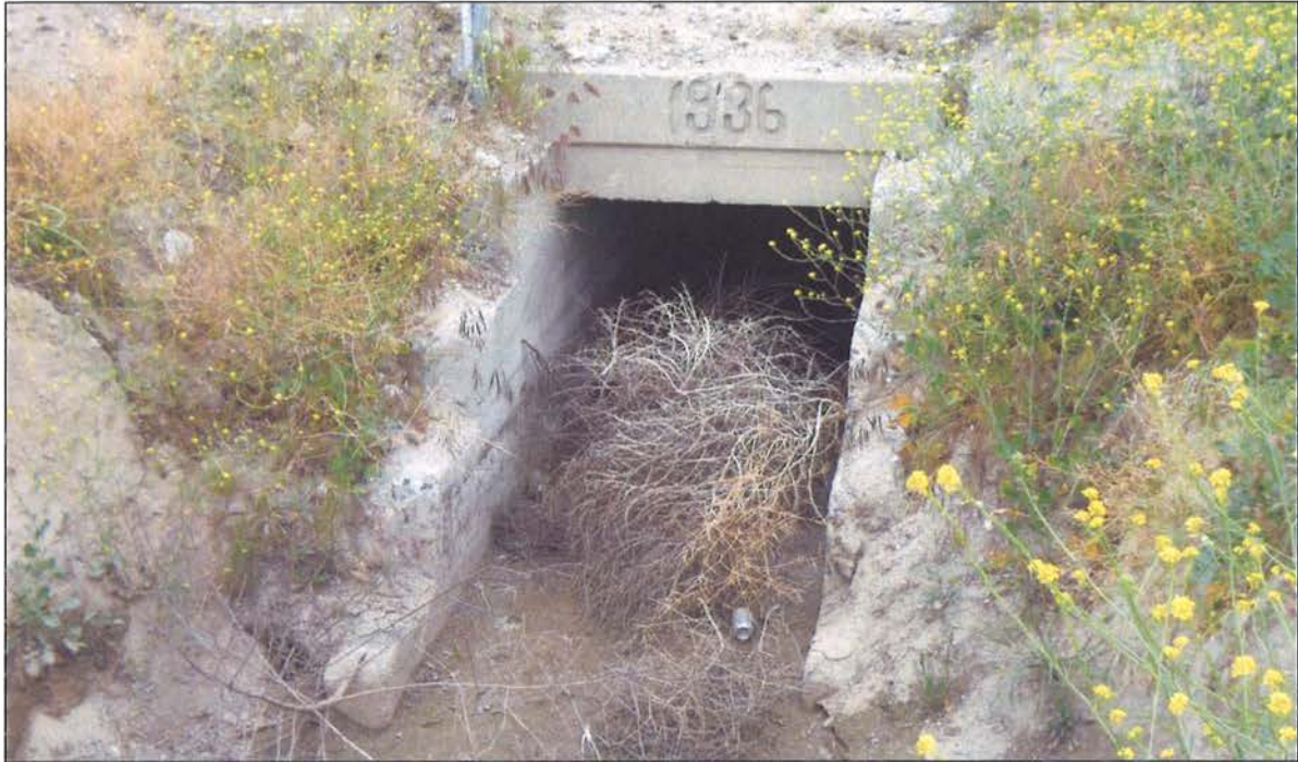
Figure 3. Culvert "B" found along Gilman Springs Road near Alessandro Boulevard (photograph taken April 25, 2012, view to the southwest). Note the 1936 date stamped on the concrete header.
