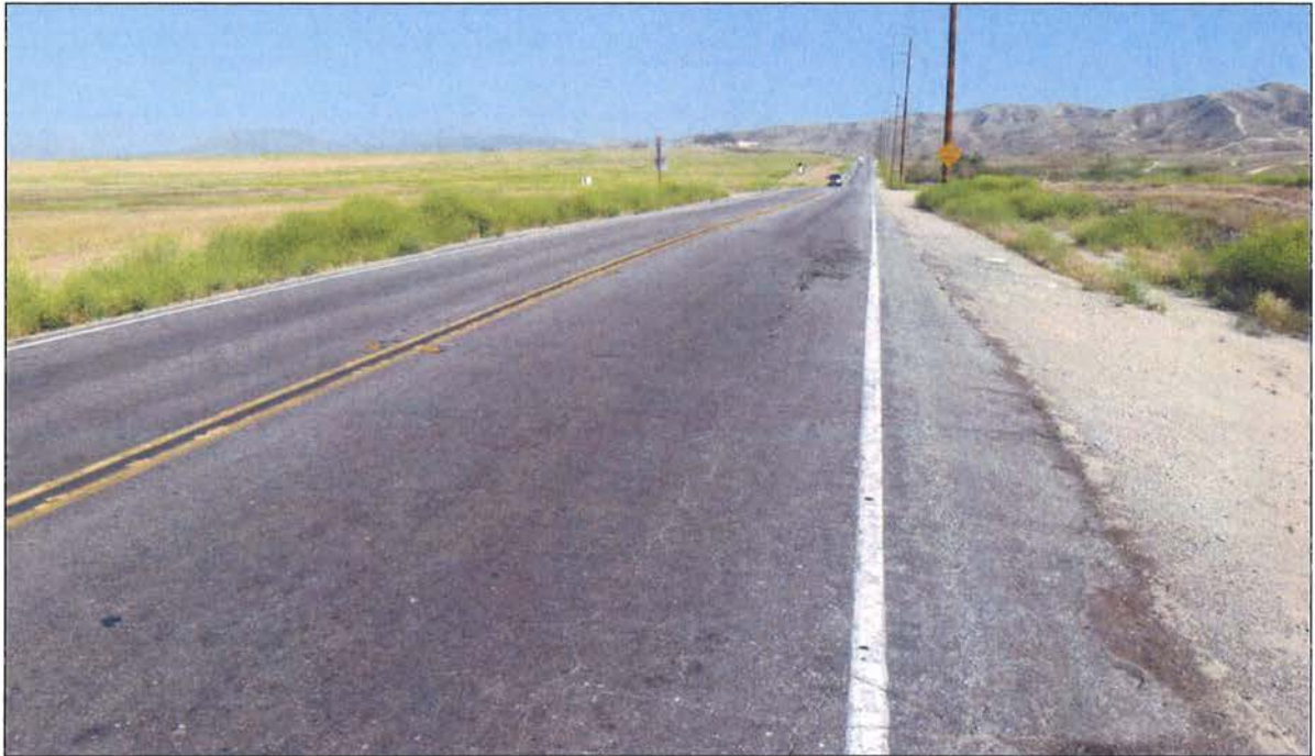
Figure 1. A segment of Gilman Springs Road in the Project APE (photograph taken May 9, 2012, view to the northwest).
