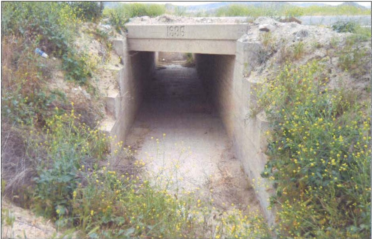
Figure 2. Culvert "A" found along Gilman Springs Road near Alessandro Boulevard (photograph taken April 25, 2012, view to the southwest). Note the 1936 date stamped on the header.
