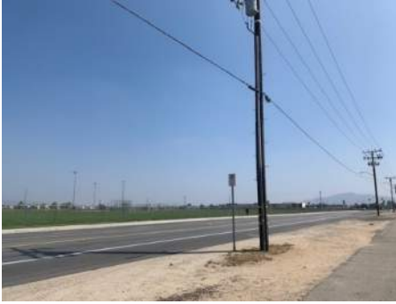
P22- Power Lines in the Northeastern Corners of the Project Site along Iris Ave.
