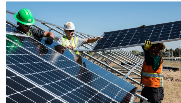
MVU and other regional and state partners offer rebates and assistance to help customers install energy efficient upgrades such as solar panels.
