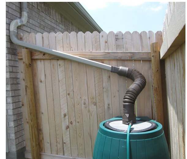
Rainwater harvesting can take the form of a greywater system (left) or a low-tech barrel in one's backyard that stores rain for a future dry day (above).
